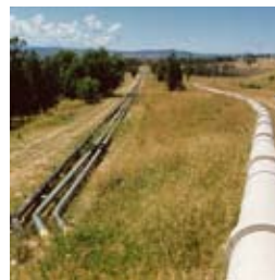
Bayswater Power Station; transporting 74% Cw fly ash slurry 11 kilometres to an abandoned open pit coal mine.
