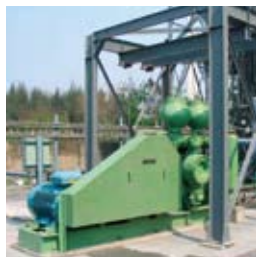
Budge Budge Power Station, India; a Geho piston diaphragm pump transports 55 m 3 /h fly ash slurry to the disposal area.
