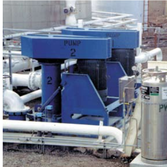
12" Warman 5000 Series pump installed in environmental containment sump
