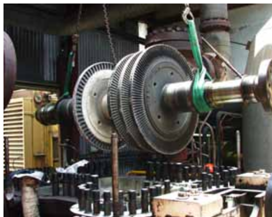
(Top) Rotors in specialist workshop at Somersby, NSW. (Centre) Dynamic balancing of rotor at Somersby. (Bottom) On-site turbine overhaul.
