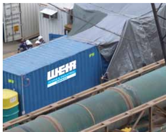
(Top) Complete overhaul of main control valve at zinc refinery by Weir Minerals Services.
