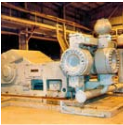
Four Geho piston diaphragm pumps transport red mud at the Alcan Gove project in Australia
