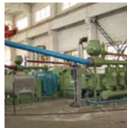
Zhongzhou Aluminum Plant, China: caustic liquor feeding
