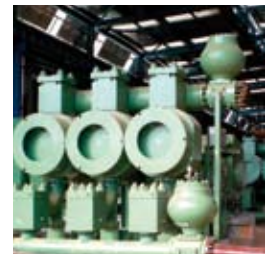
Paragominas, Brazil: long distance bauxite slurry pipeline transportation
