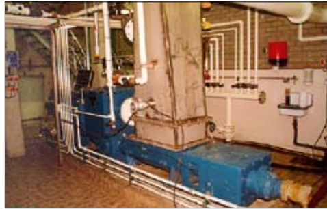
RWZI Dordrecht, the Netherlands: sewage sludge transport
