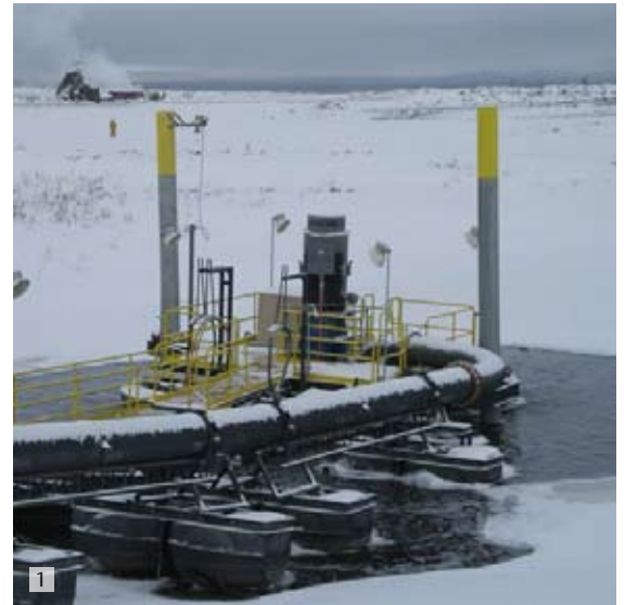
1 : Hazleton vertical cantilever with 800HP motor on 11' pontoon
