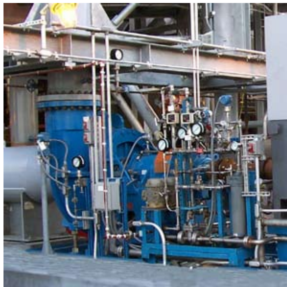
Below right: Coke fines vertical slurry pumps
