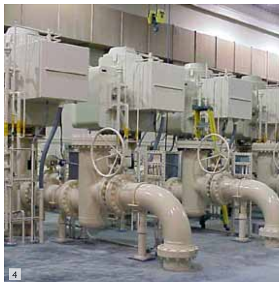
1: Booster pumps 2: High service pumps 3: Sump pumps 4: Booster pumps
